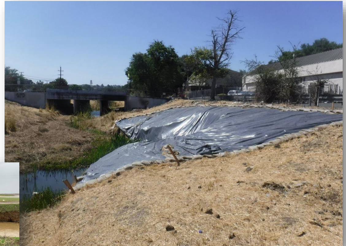
Invasive vegetation and bank erosion
