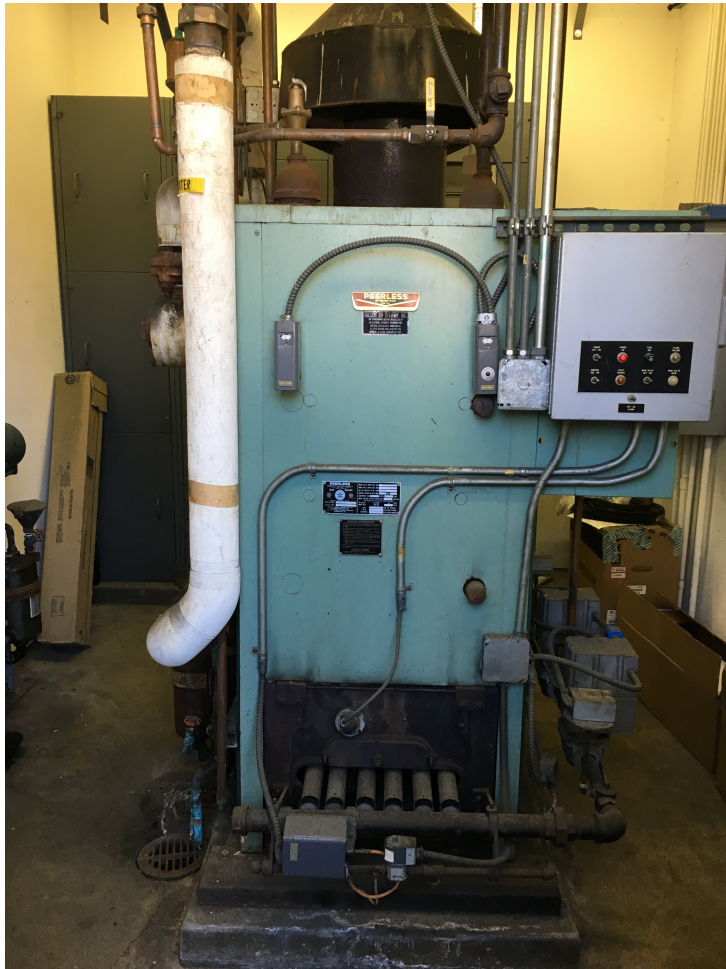
48-year-old boiler at Fire District Headquarters has far exceeded operational life expectancy
