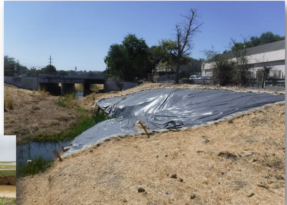
Invasive vegetation and bank erosion
