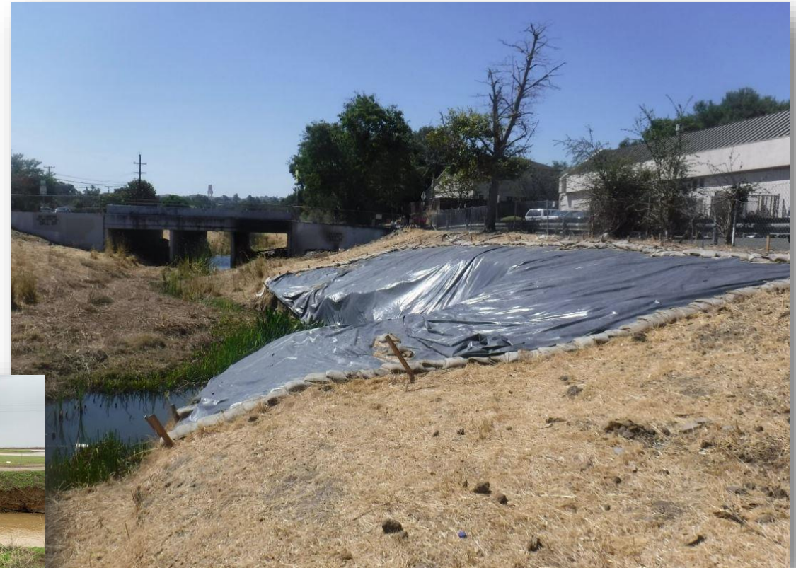
Invasive vegetation and bank erosion
