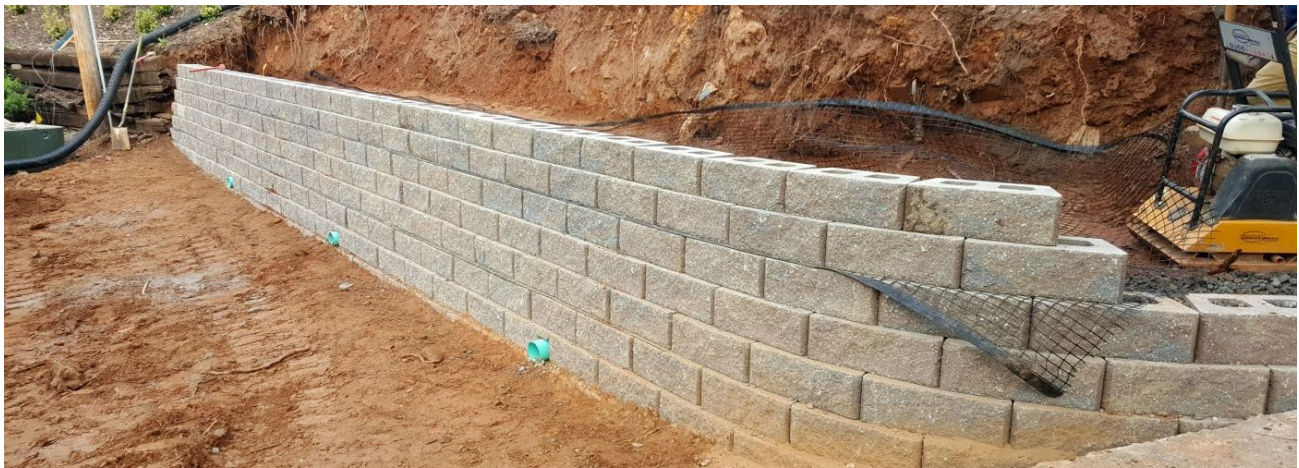
Figure 4-18. Concrete masonry unit retaining wall (could be covered with soil and planted on
