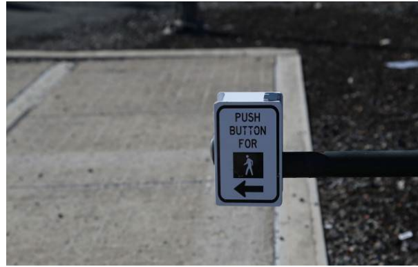
Existing pedestrian signal button at crosswalk of Marina Vista Way.
