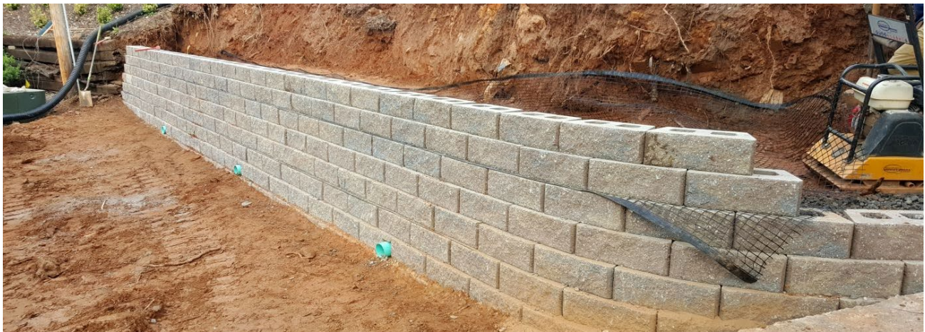
Figure 4-18. Concrete masonry unit retaining wall (could be covered with soil and planted on
