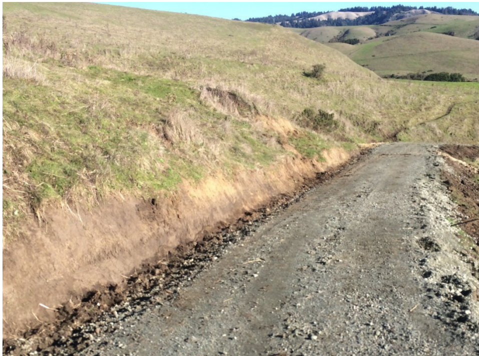
Figure 4-12. Lime-treated base rock surface after use and weathering
