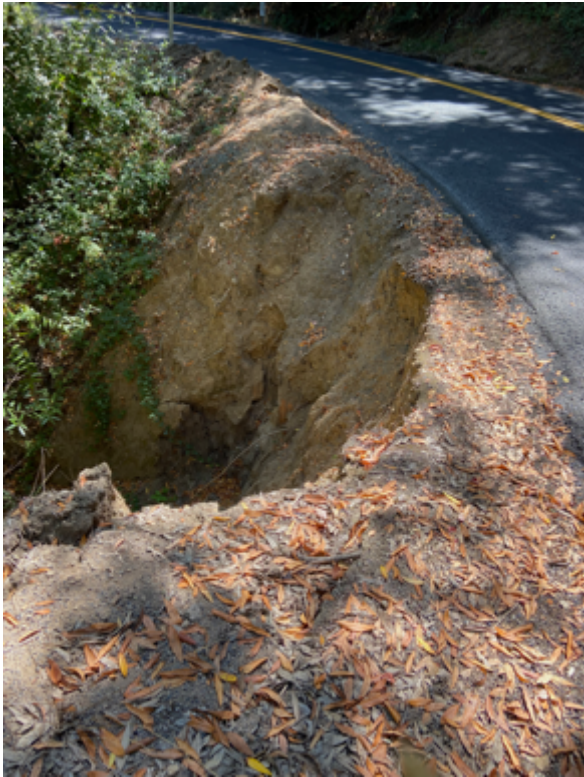
Repair Location 3 – postmile 4.6-4.7. Culvert washout undermining road. Replace culvert and establish erosion control such as gabion baskets or interlocking concrete bars, and guardrail.
