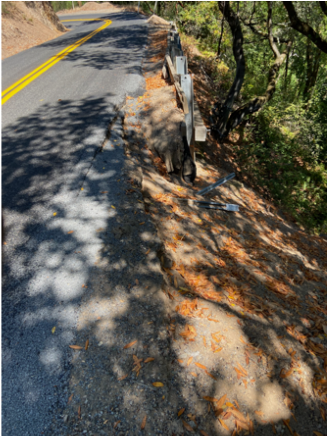
Repair location 4 – postmile 4.3 Earlier repair that needs new wood and extension to cover undermining shoulder.
