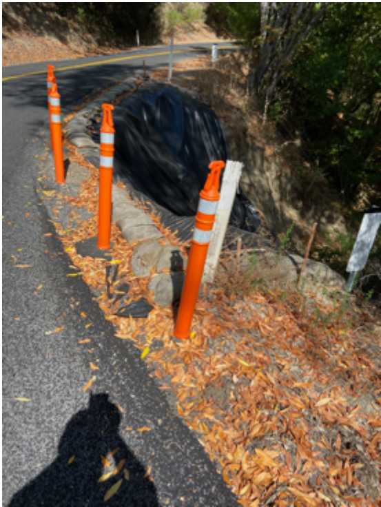
Repair Location 1 - On Pinehurst Road near postmile 0.2 there is a culvert washout needing repair with possibly a gabion wall, or interlocking concrete bars or some other form of structural support and possible culvert replacement.
