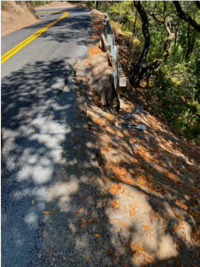
Repair location 4 – postmile 4.3 Earlier repair that needs new wood and extension to cover undermining shoulder.
