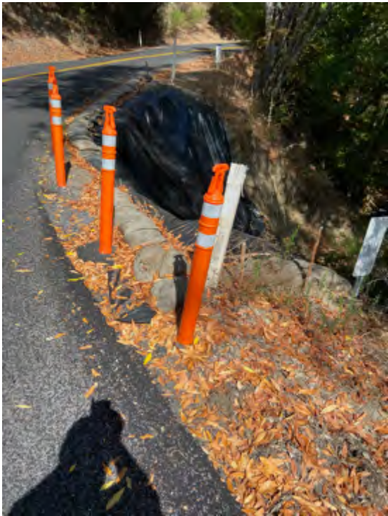
Repair Location 1 - On Pinehurst Road near postmile 0.2 there is a culvert washout needing repair with possibly a gabion wall, or interlocking concrete bars or some other form of structural support and possible culvert replacement.
