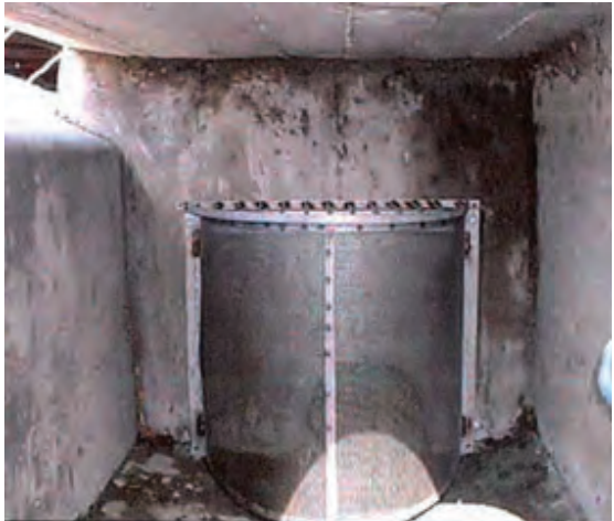
Inside of a drainage inlet retrofitted with a trash capture device.
