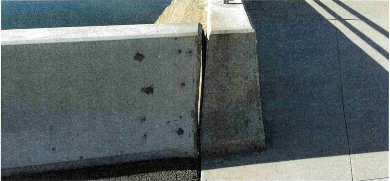
Photo 6 – Separation in parapet wall where asphalt and concrete meet on dam crest.
