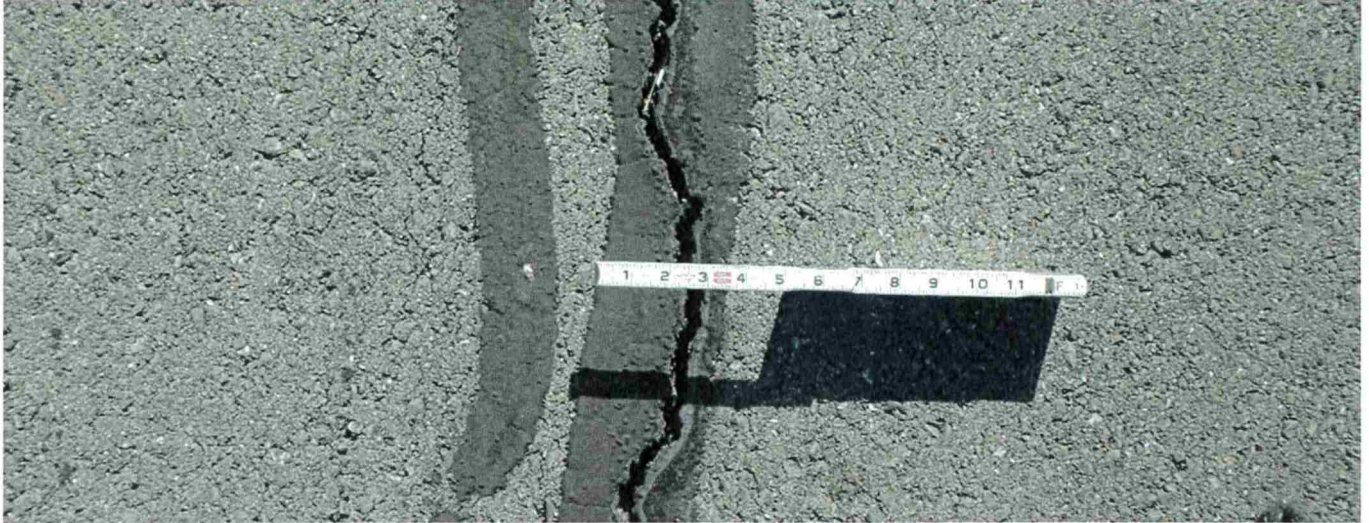
Photo 4 – Close-up of longitudinal crack on left side of dam along asphalt crest.
