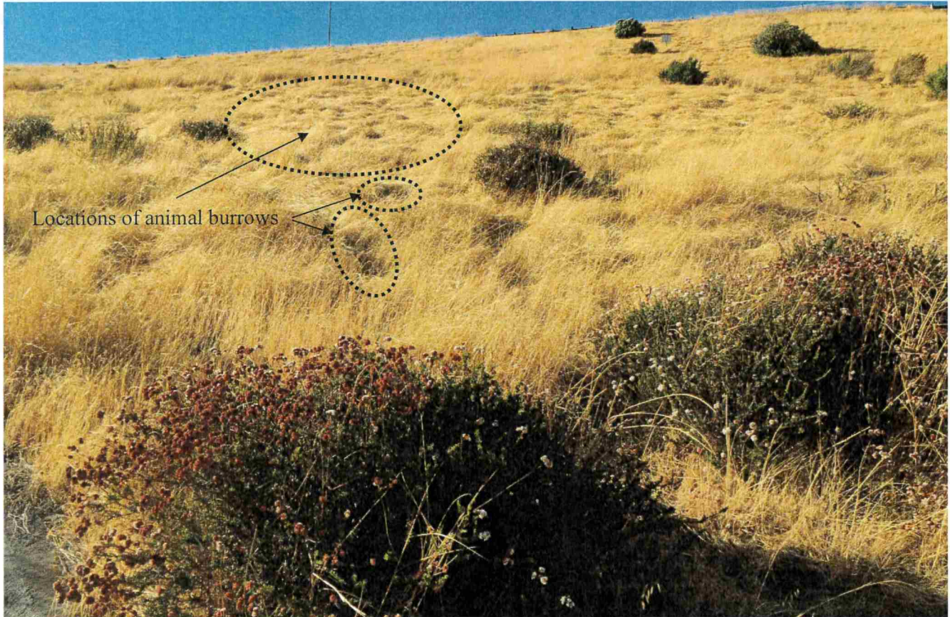
Photo 2 – View of downstream slope taken from V-channel on right side of dam showing slope vegetation and animal burrows.
