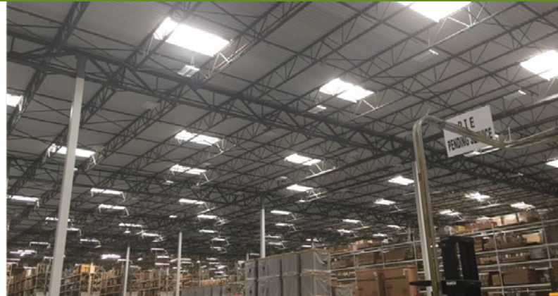
PHOTO: A combination of natural and LED lights provide the right mix of lighting sources
