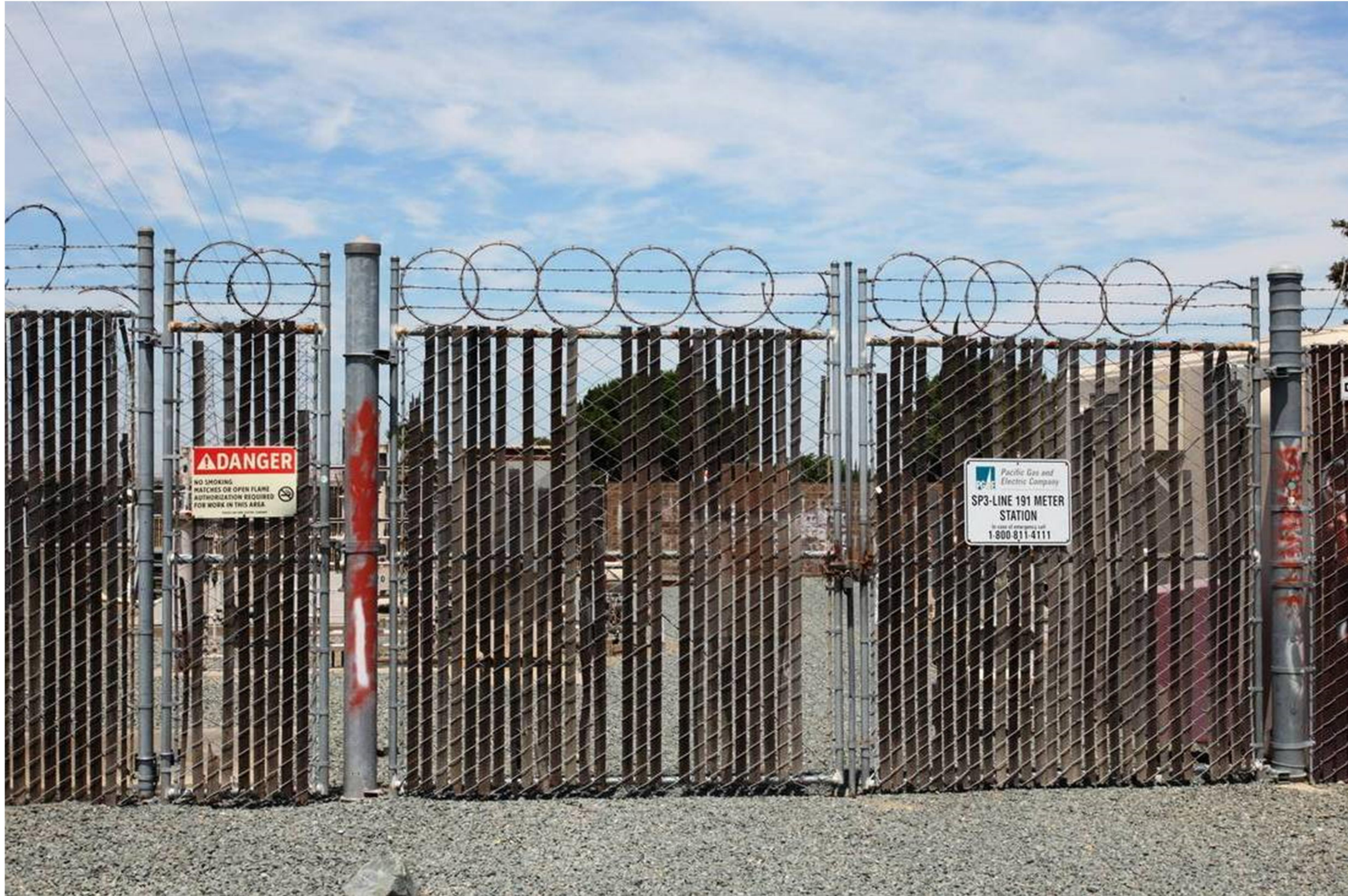
Figure 15 (continued) PG&E STANPAC3 Facility Looking North
