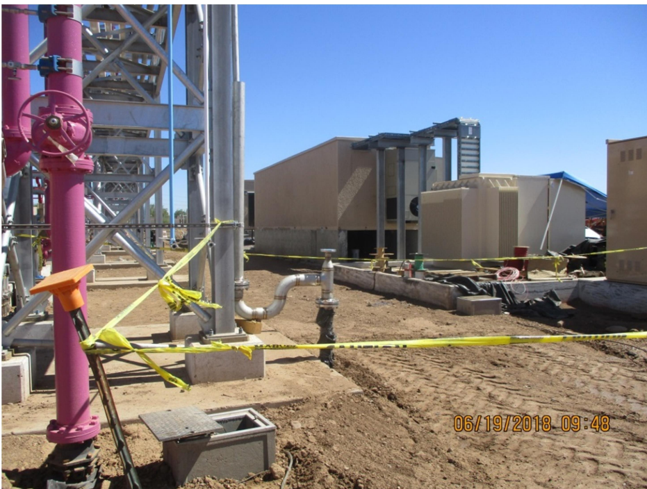
Overhead Pipe Assembly (left); Control Center on Skid (center)
