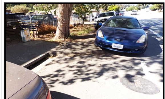
Concrete Sidewalk terminates at tree. Inadequate pedestrian facilities with cars parking on path in Segment 2.
