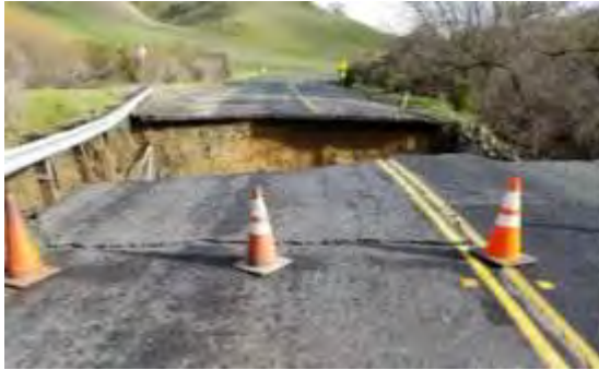
Figure 11: Washout of Alhambra Valley Road in West County
