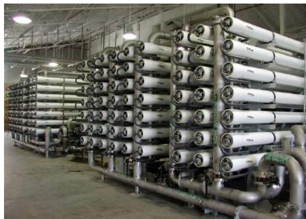
The 5-MGD Newark Desalination Facility uses reverse osmosis for groundwater desalination.
