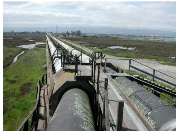
The Bay Area is home to aging water, wastewater, stormwater, and flood protection infrastructure.
