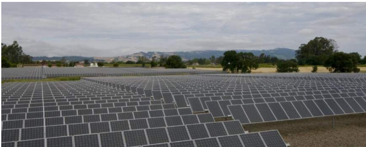
Sonoma Valley Wastewater Treatment Plant Solar Panels
