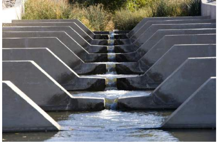
An example of a fish ladder installed as to aid fish passage on a Bay Area stream.
