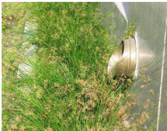
An interior roof drain discharges to a vegetated swale in Emeryville, CA. This is an example of an “approved alternate location” for stormwater discharge. From SFPUC, 2009.
