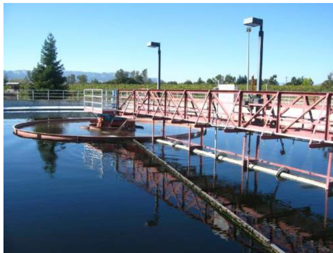
Sonoma Valley Wastewater Treatment Plant, Clarifier
