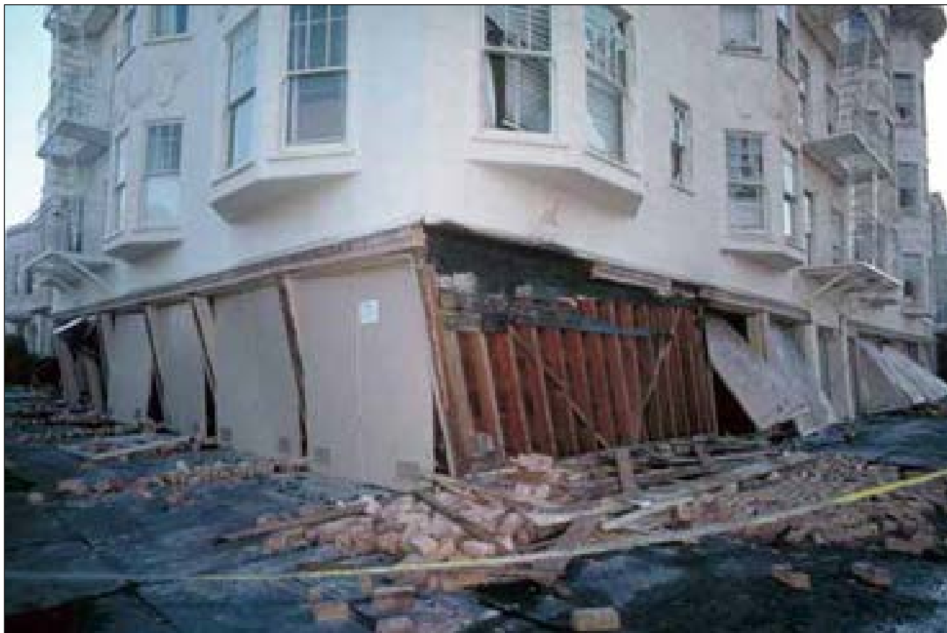
Figure 8-12. Soft-Story Damage from 1989 Loma Prieta Earthquake
