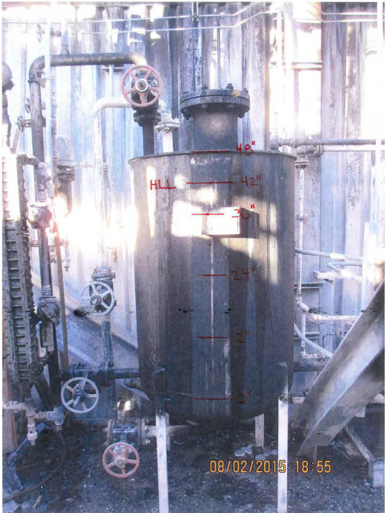
PICTURE OF DAY TANK WITH LEVELS MARKED
