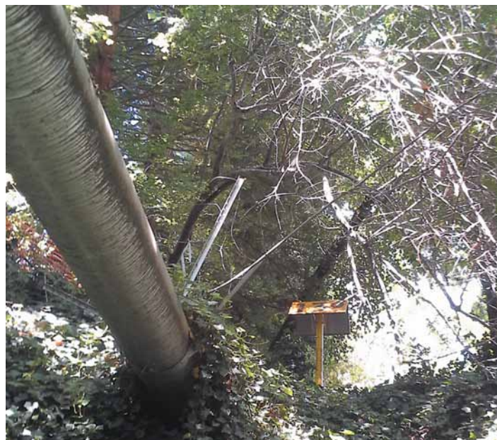
The San Jose line inside protective sleeve traveling above ground across a seasonal stream along the Iron Horse Corridor.
