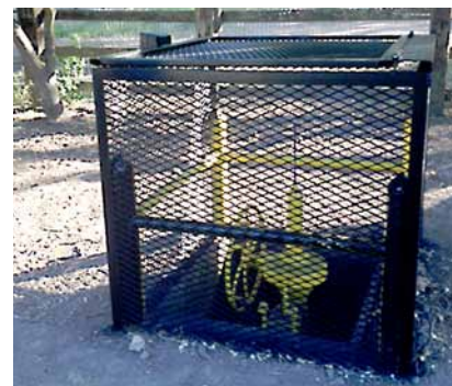
Manual valve inside protective cage in Alamo along Iron Horse Corridor
