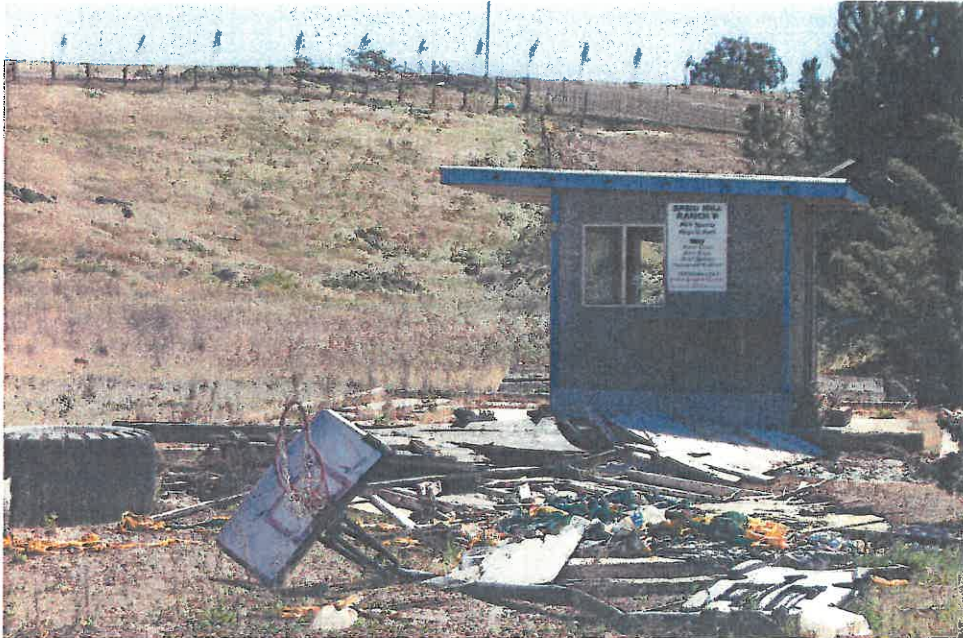
Track area (before cleanup), showing trash and vandalism.
