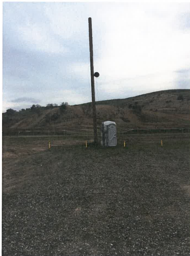
Figure 4: Existing PA Loudspeaker on Pole at SW Corner of Parking Lot
