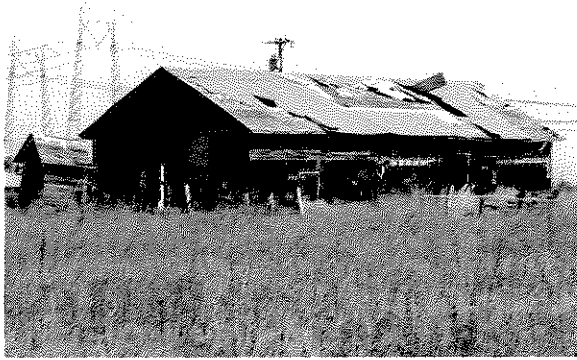
Barn in Disrepair
